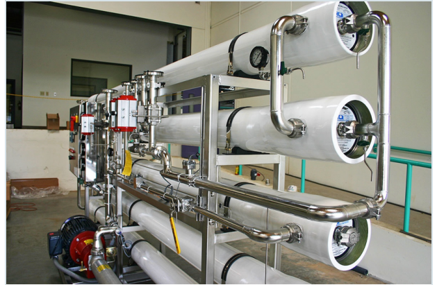
EPS biofouling on RO membrane skids raises pressure drop and cuts flux long before scale does.
