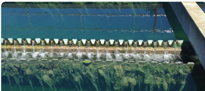
BEFORE — algae overgrown on the clarifier weirs.
